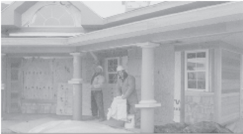
COMING SOON - Workman Jim Dimitrievski and foreman Jim Huxford stuff insulation into the portico of OB-GYN's new Arrowood Drive home in Lansing's Parkview Health Care Campus next to Convenient Care off Warren Rd.
