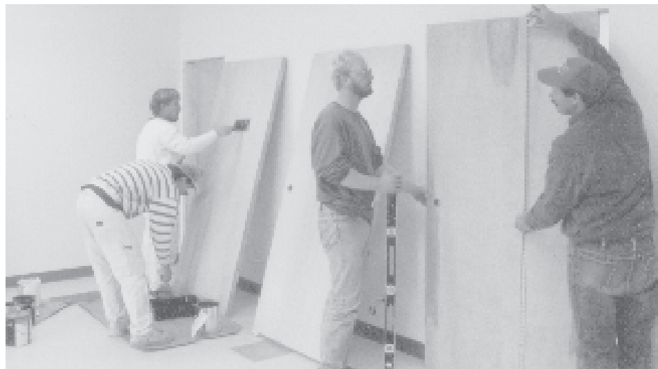
HANGING TEN (or 20) doors is no big deal for artisans Skip Percey, Steele Steffy, Mark Barber and Greg Koski as they put the finishing touches on the new Ithaca Montessori School on Ascot Place in Lansing Village before the November 8-11 moving days.
